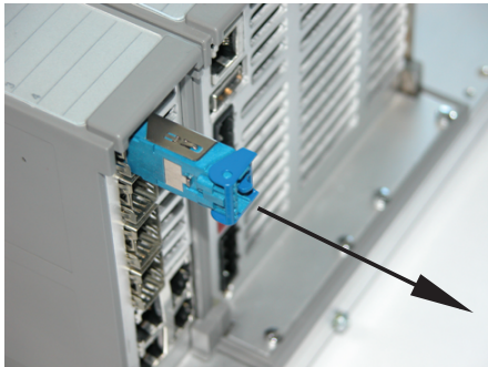
Figure 19: Deinstalling an SFP module
